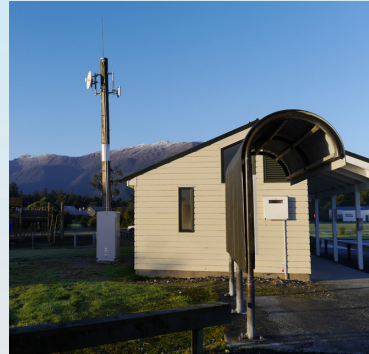
The repeater installed at Haast Township.
