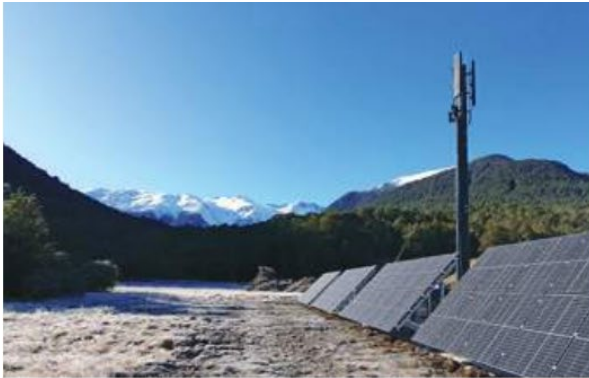
Tower at Mirror Lake, SH94, showing the solar panels for the off-grid power supply
